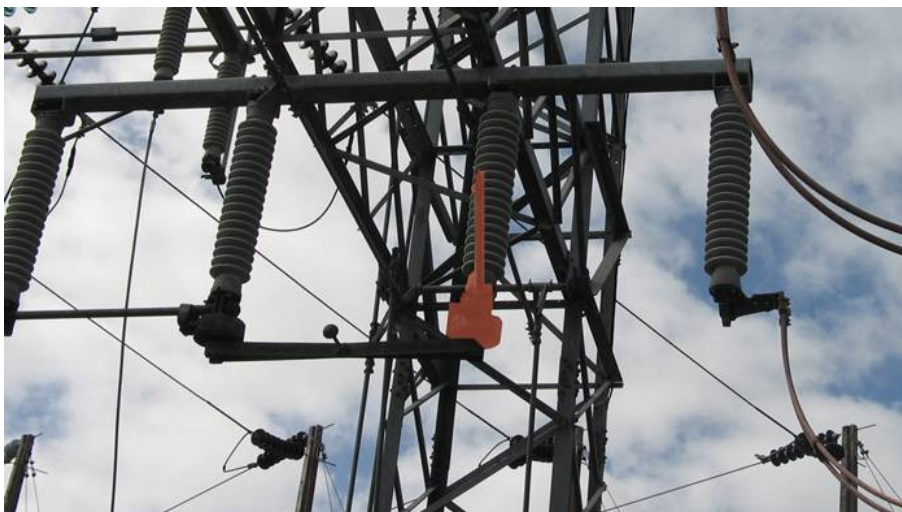
Example of an open disconnect switch.
