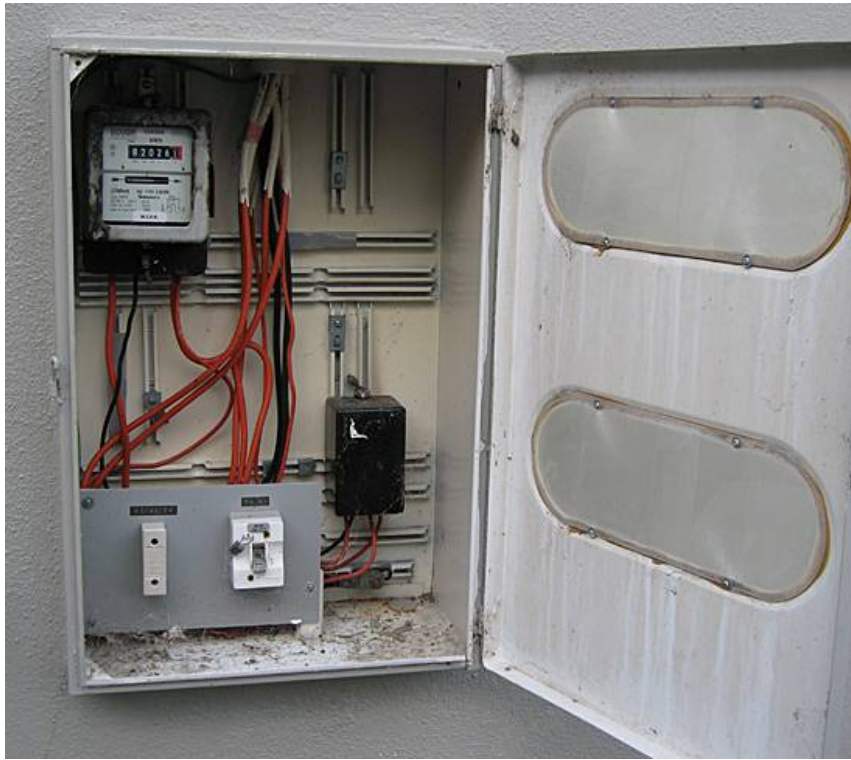
Electricity meter measuring electricity usage.
